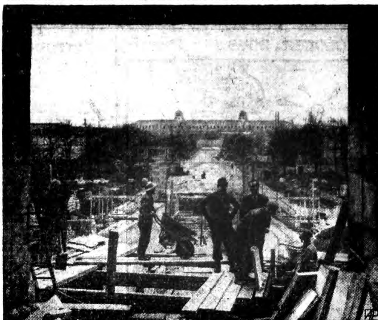
BUILDING OLYMPICS ROAD — German prisoners of war help British workmen build a new approach road to Wembley Stadium (background) for the 1948 Olympic games.
